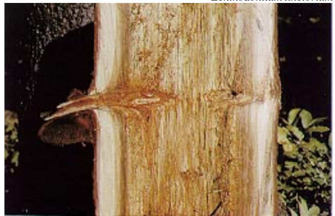
Typical rot caused by Echinodontium tinctorium
