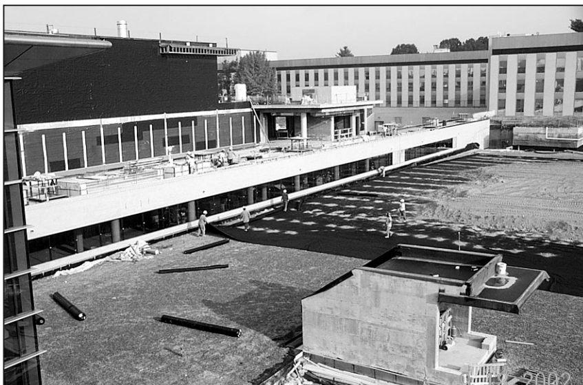
NIST's Advanced Measurement Laboratory, now under construction, will be one of the most advanced research buildings in the world when occupied in 2004.
