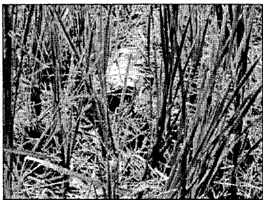
This is a well hidden outlet.
