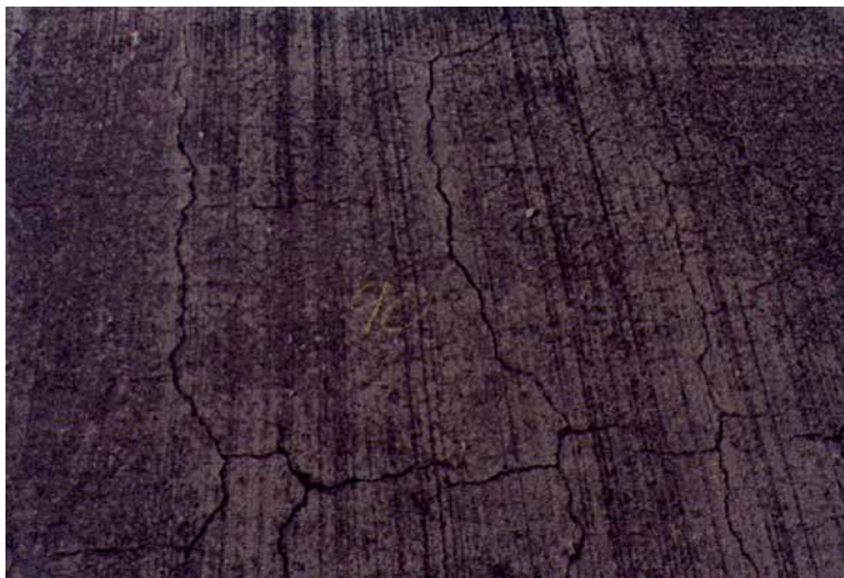
Figure 40. Close-up photograph showing typical map cracking (Boron, CA).
