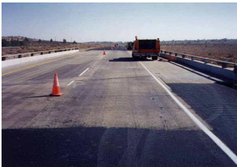
Figure 35. Treated section on Boron overhead structure over State Route 58 looking east (Boron, CA).
