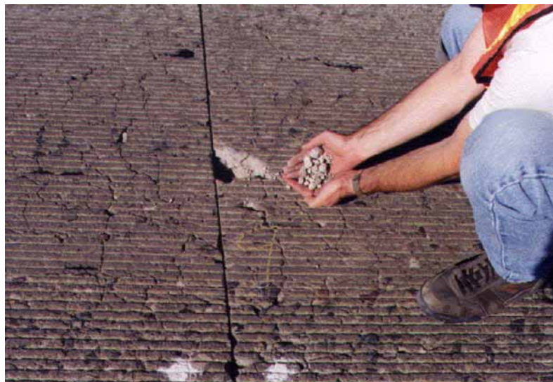
Figure 46. Photograph showing an example of high-severity joint distress (Boron, CA).
