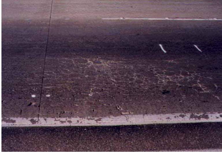
Figure 39. Example of high-severity map cracking (Boron, CA).
