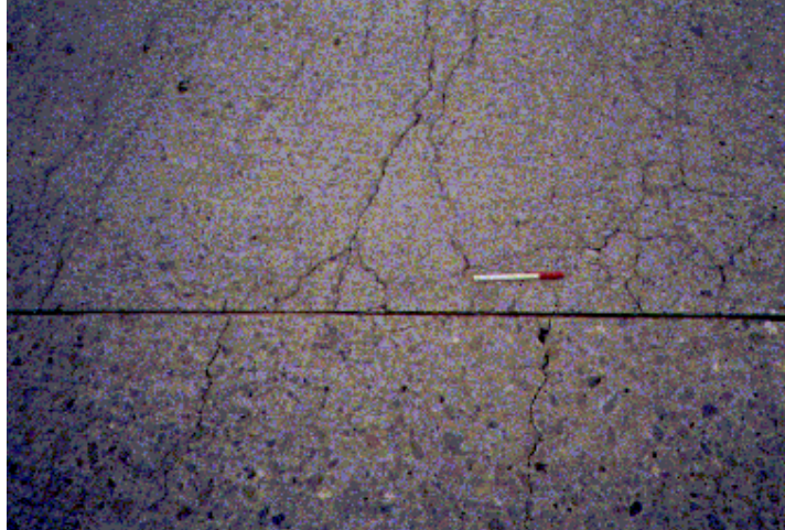
Figure 4. Joint distress of medium severity (Winnemucca, NV).
