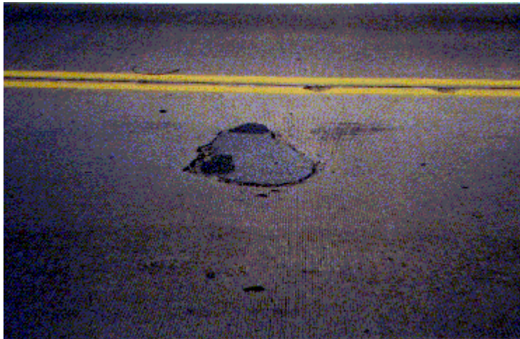
Figure 28. Asphalt patch in center of section in travel lane (Newark, DE).
