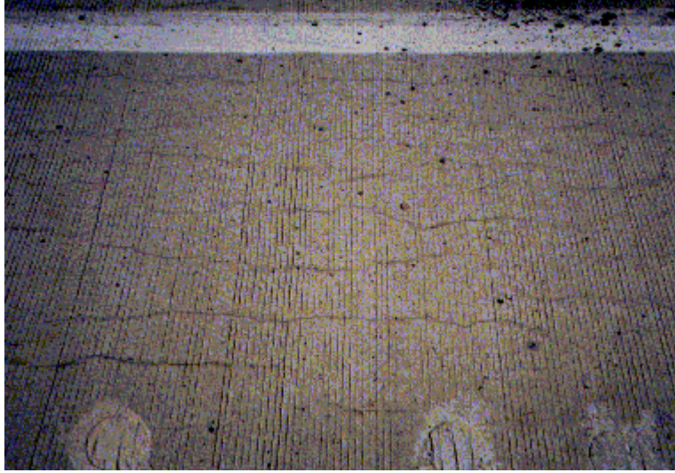
Figure 23. Typical longitudinal cracking (Newark, DE).
