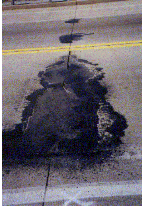
Figure 27. Asphalt concrete patching along transverse joint in travel lane (Newark, DE).
