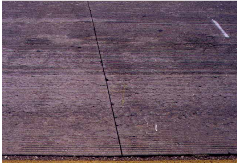
Figure 45. Photograph showing medium-severity joint distress (Boron, CA).
