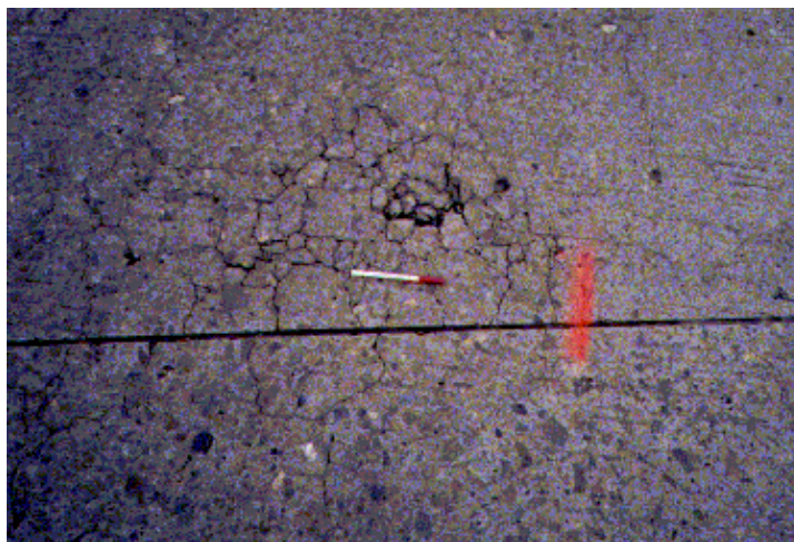
Figure 3. Joint distress of high severity (Winnemucca, NV).
