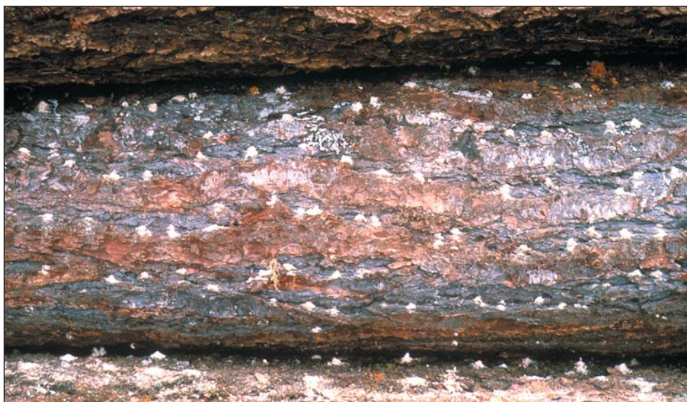
Piles of white boring dust indicate ambrosia beetle attacks
