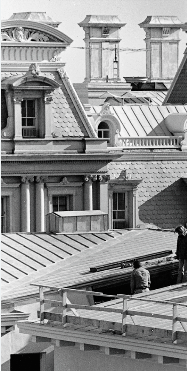
Workmen on the roof of the Winder Building, Washington, D.C. install a window as part of a renovation project.
