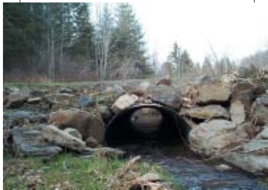
A pipe-arch culvert used on a tributary of Clear Creek eight miles south of Estacada is one example of responsible riparian management under the Oregon Plan for Salmon and Watersheds. The landowner is Port Blakely Tree Farm.
