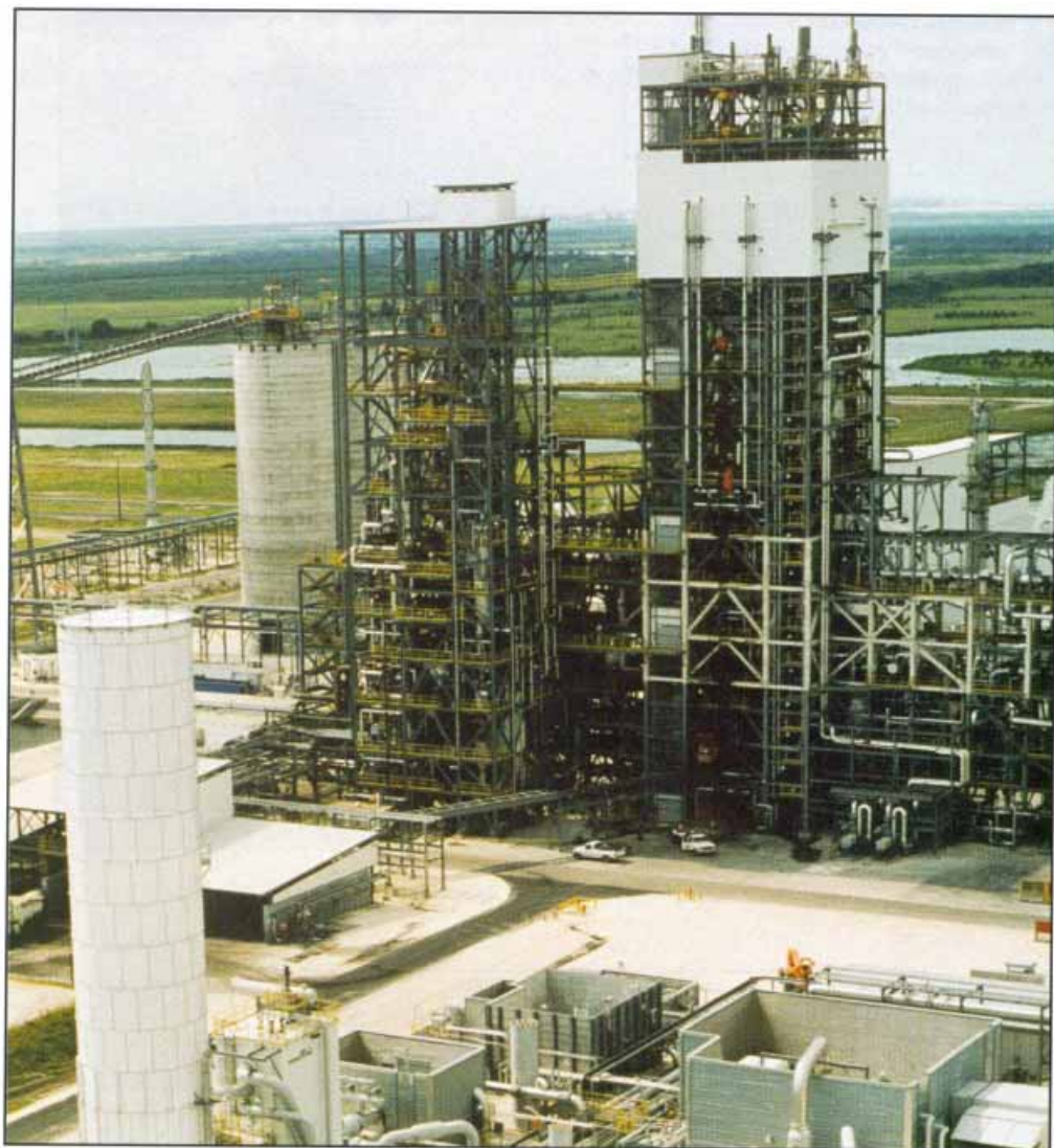
The Texaco gasifier is in the largest structure, which also contains the radiant syngas cooler. The hot gas cleanup system is installed in the smaller of the two large structures. In the foreground is the air separation unit.
