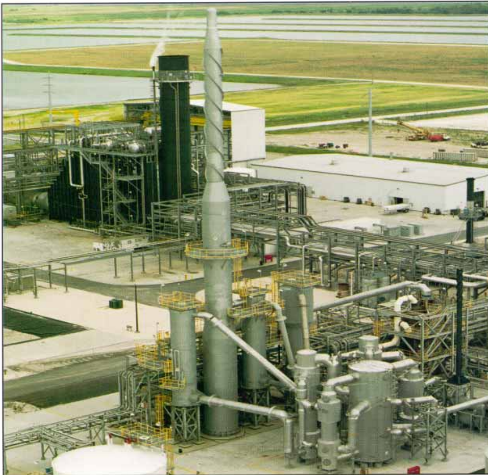
The sulfuric acid plant is in the foreground and the combined-cycle unit is in the background. The large black object (left center) is the heat recovery steam generator.
