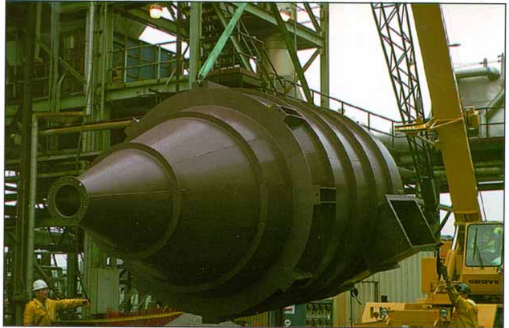
The cyclone is being moved to the layout area for insulation prior to installation.
