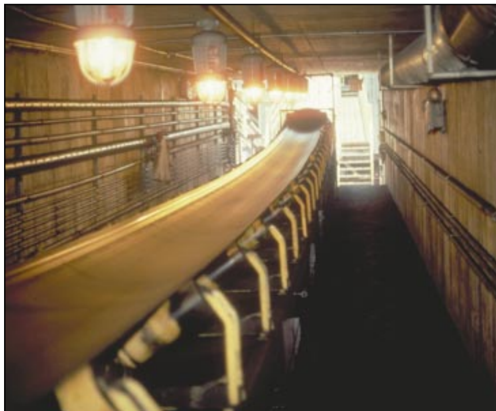
Raw coal conveyor belt
