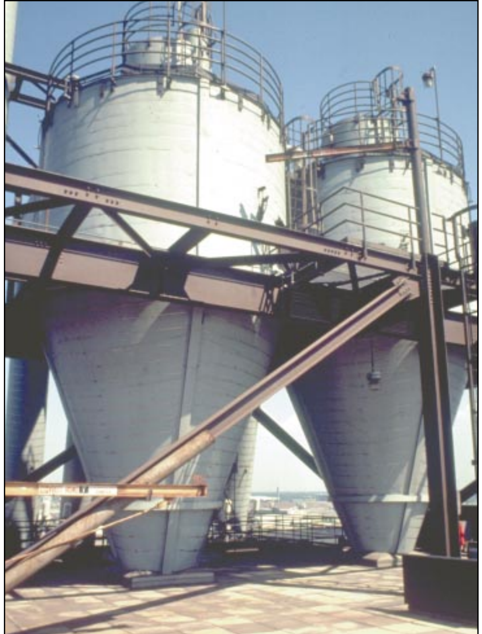
Cyclone separators on coal grinding mills
