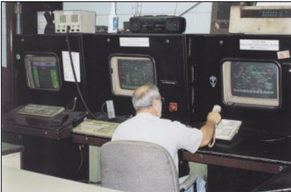
Granulated coal injection control room
