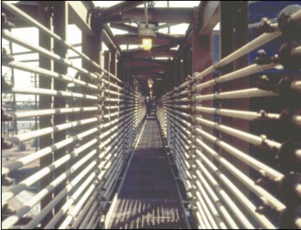
Transport piping to carry coal from preparation area to tuyeres
