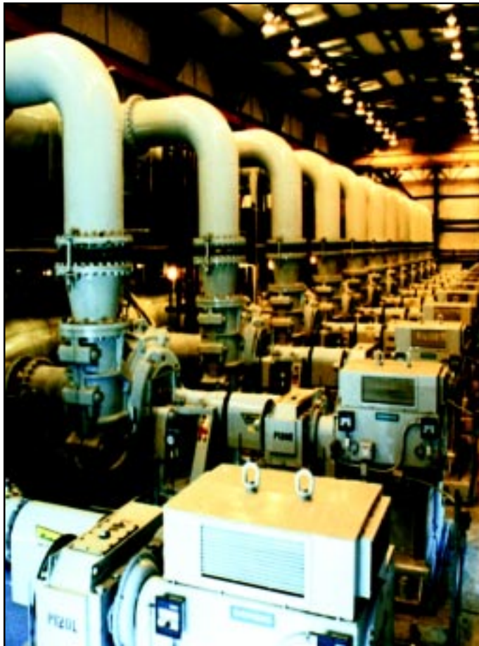
Sorbent recirculation system at Bailly Station.
