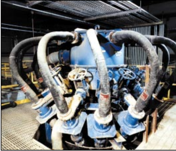
Hydrocyclone in gypsum dewatering system at Milliken Station.
