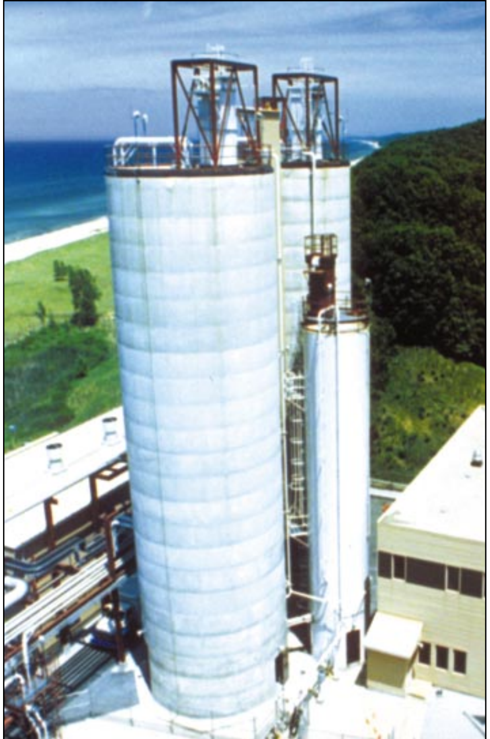
Limestone and lime silos for AFGD Demonstration Project, adjacent to Indiana Dunes National Lakeshore.
