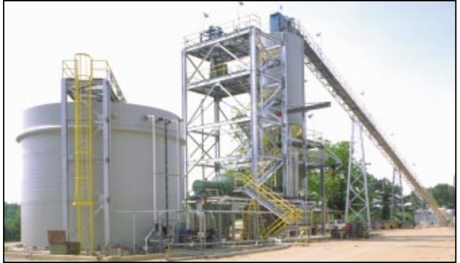
Limestone unloading conveyor, slurry tank, and hopper at CT-121 Demonstration Unit.
