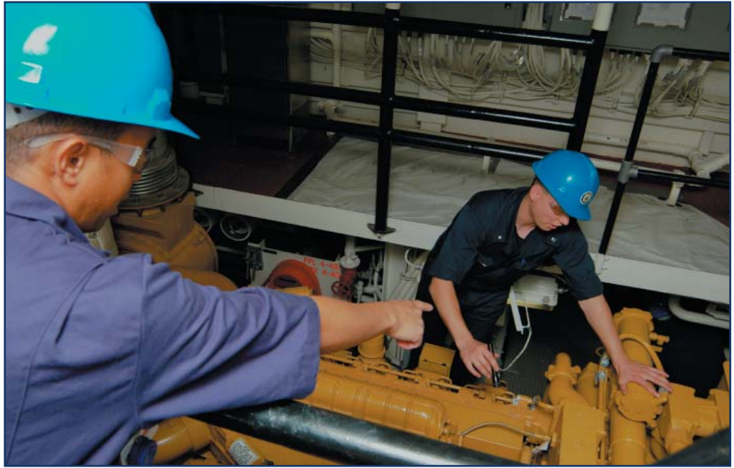
PASCAGOULA, Miss.—Petty Officer 1st Class Demosthenes Daniel, an electrician’s mate, shows Petty Officer 3rd Class Adam Novotny, a machinery technician, parts of the first National Security Cutter’s ship service diesel generator set. BERTHOLF has three diesel generators that can be aligned to provide primary, standby and emergency power. (USCG photo by Petty Officer 3rd Class Michael Anderson)
