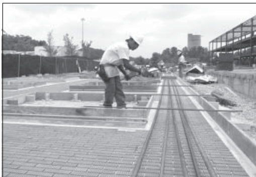
The privately funded facilities' walls are built flat on the ground (above) and raised by cranes.
