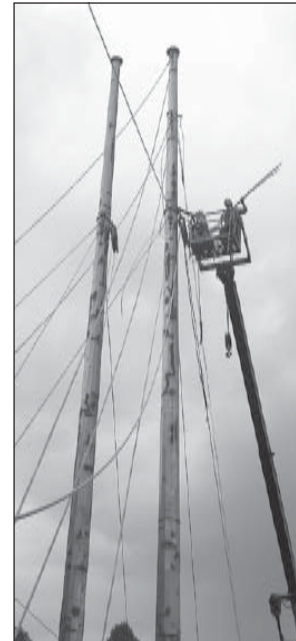
Workmen install support towers for the conductor tests near Bethel Valley Road.
