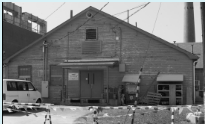
Building 3550’s “flaky” exterior
