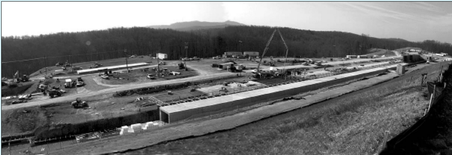
A recent shot of the SNS construction site. The Earth's curvature is factored into the construction of the linac tunnel, shown in the foreground.
