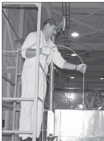
Stan Cooper of the M&C Division is installing a lift device for a U-233 canister.
