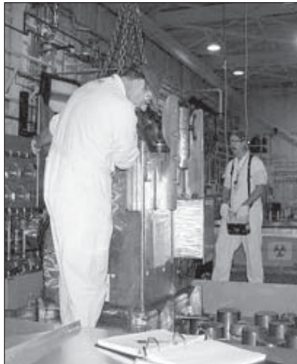
Stan Cooper (left) and Karl Thomas of Nonreactor Nuclear Facilities Division are installing the inspection chamber above the tube vault
