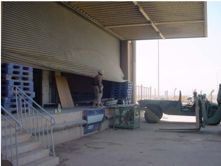
Damaged Roller Doors – Truck Docking Station
