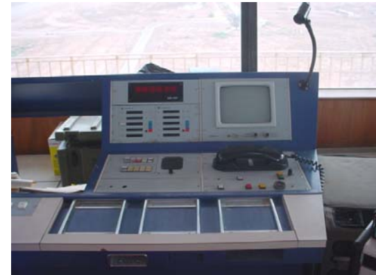
ATC Consoles – Communications
