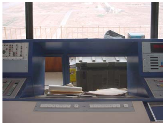
ATC Consoles – Missing Radar Display
