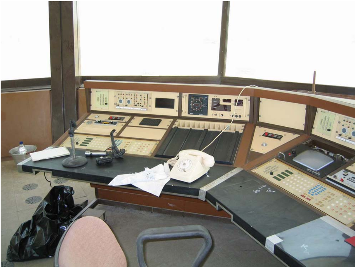
Control tower - consoles
