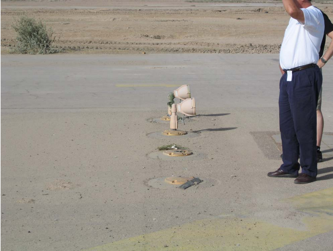
Damaged approach light fixtures
