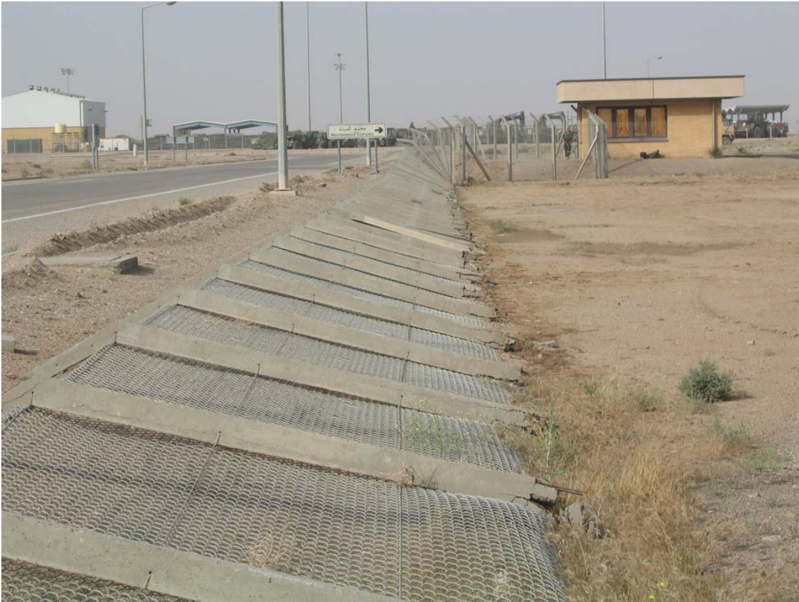
Security fence posts damaged by salt attack
