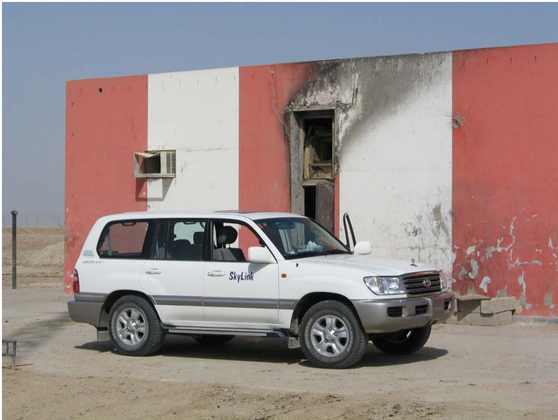
Damaged transmitter building
