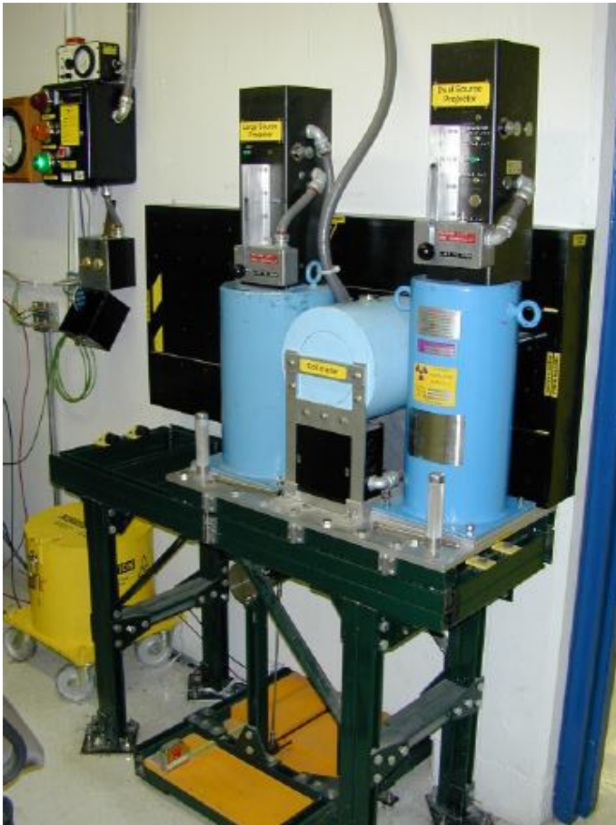
Cylindrical Collimator Located in Center that Required Manual Insertion of Wand-Type Sources
