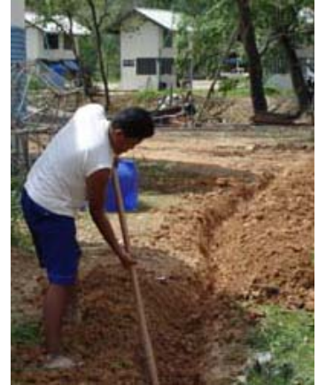
Villagers dig trenches for pipelines to connect their homes to the new water system. Photo: USAID/Chris Dunbar
