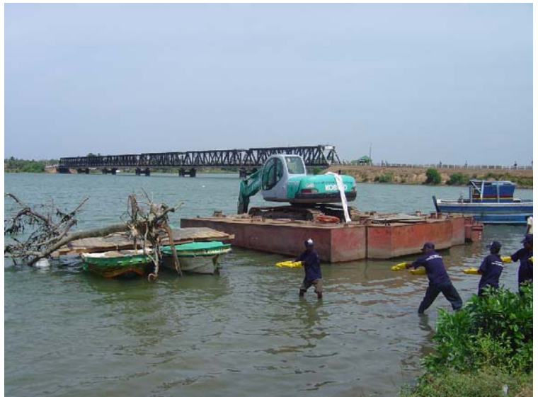
Workers remove a felled tree from the lagoon at Batticaloa while executing the USAID project.
