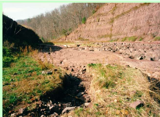
Fig. 2.3-12 Spillway damage, Switzer Dam, Dry River, VA
