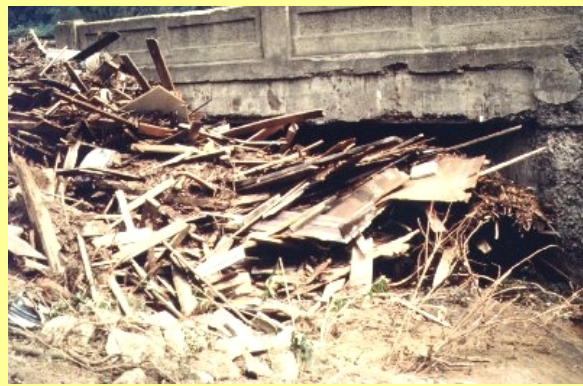
Fig. 2.3-1 Debris blockage of a bridge
