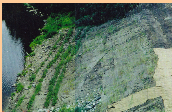
Fig. 2.3-9 Composite photo, live plantings in rock base (left) and soil bioengineering using geotextiles, Glen Arbor, Santa Cruz Co., CA
