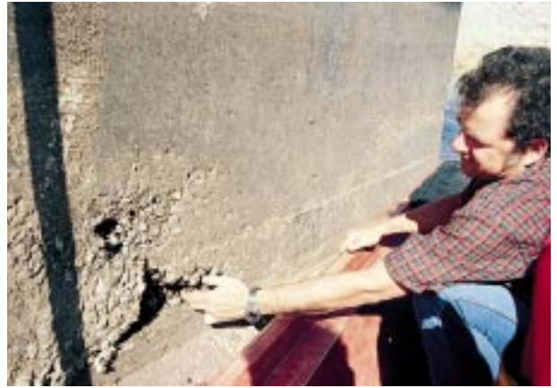
Concrete principal spillways and pipes on many of the older upstream flood control dams are beginning to deteriorate and will need replacing to ensure safety of the dam.
