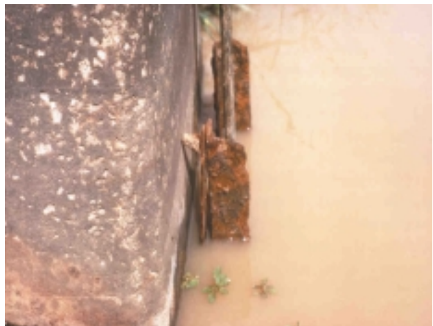
Figure 6 Deterioration of Metal Slide Gates in Dams
