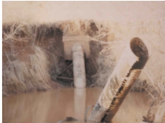
Figure 5 Deterioration of Metal Pipes in Dams
