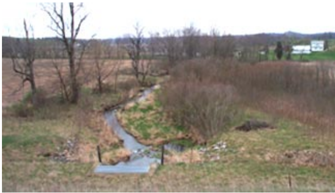
Looking downstream from back of dam. Homes are located in the flood plain below the dam.
