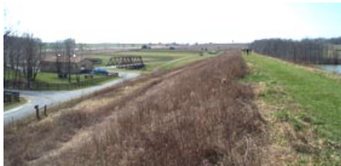
Rush Creek 7C dam is in good condition, but due to development downstream it no longer meets dam safety requirements.
