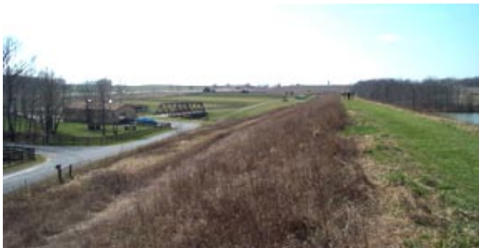
The dam protects homes, roads and other structures including Interstate highway 76, which would be at risk if the dam failed.
