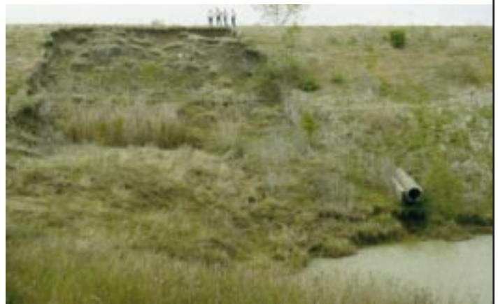
Unstable slopes on earth dams is a major problem.
