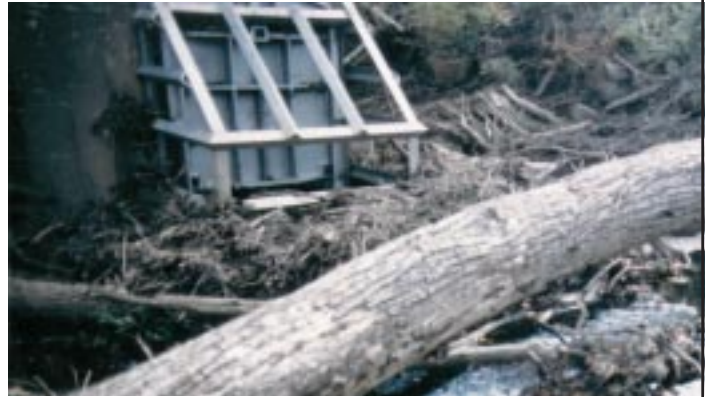
TYPICAL PROBLEMS. Damaged trash racks or gates prevent proper operation of the reservoir. Large amounts of debris and sinkholes, shown here at the outlet, can result.
