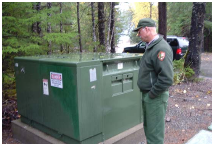
Photo 3: Modular Oil Switching Terminal (MOST) #5 located at east end of Bartlett Cove electric distribution system.
