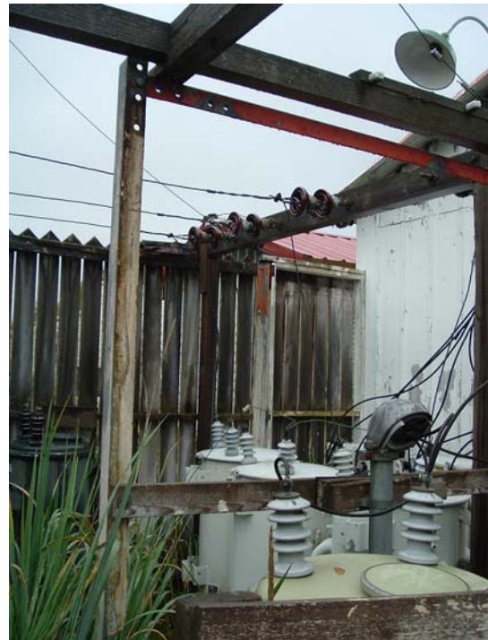
Photo 4: Portion of GEC transformer yard at the powerhouse.
