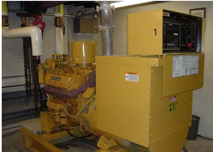
Photo 1: Diesel generator Unit No. 1 at Bartlett Cove.
