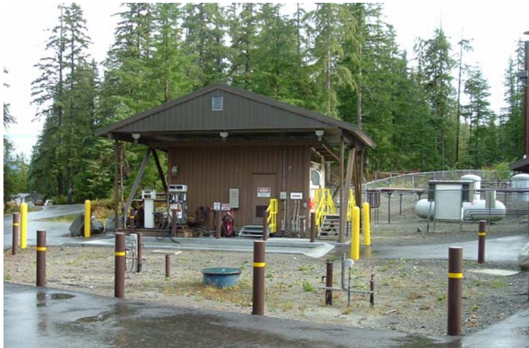
Photo 2: Fuel dock and underground fuel storage facility near the utility service building at Bartlett Cove.
