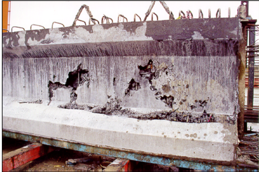
Figure 1. Honeycombing in Girder B-4
