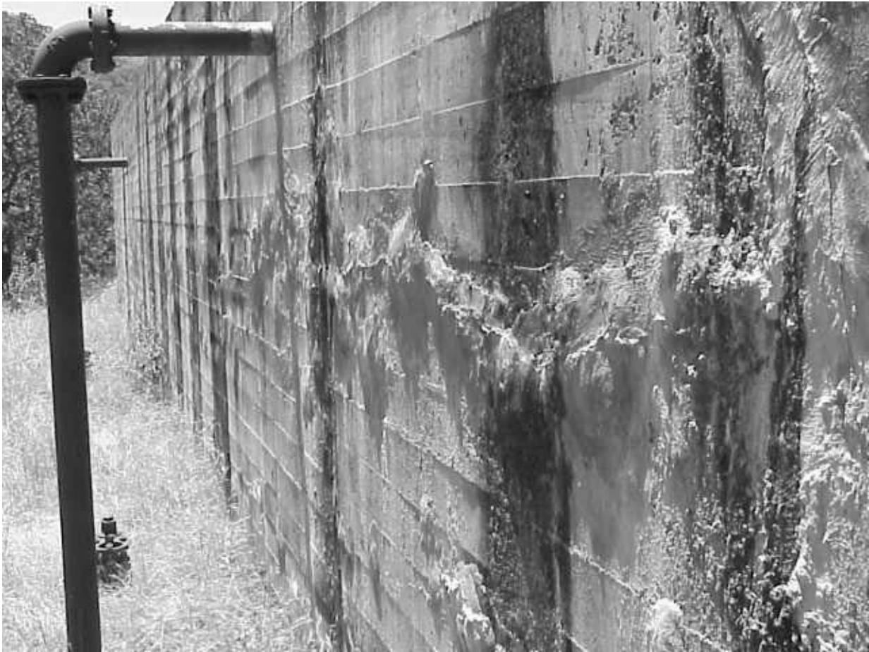
FIGURE 9. VISIBLE TANK CRACKS AND WATER LEAKAGE
