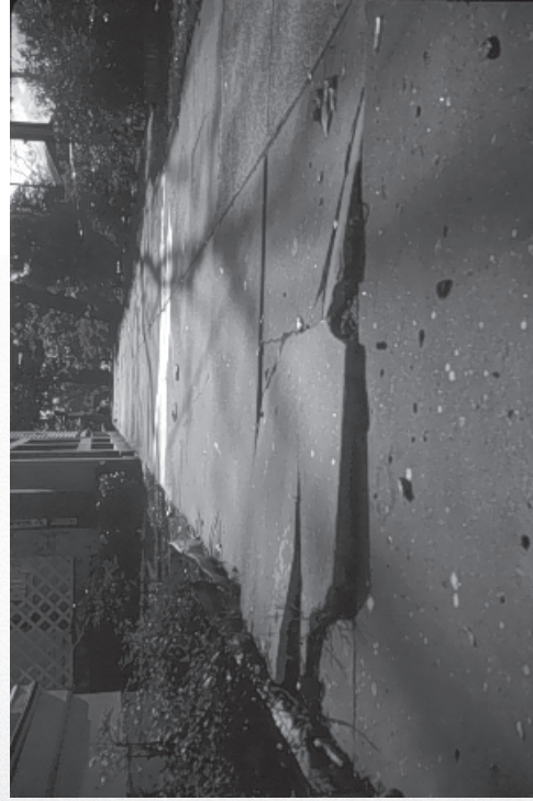
Figure 10-1. Regular sidewalk maintenance can prevent or correct sidewalk conditions, such as changes in level.
