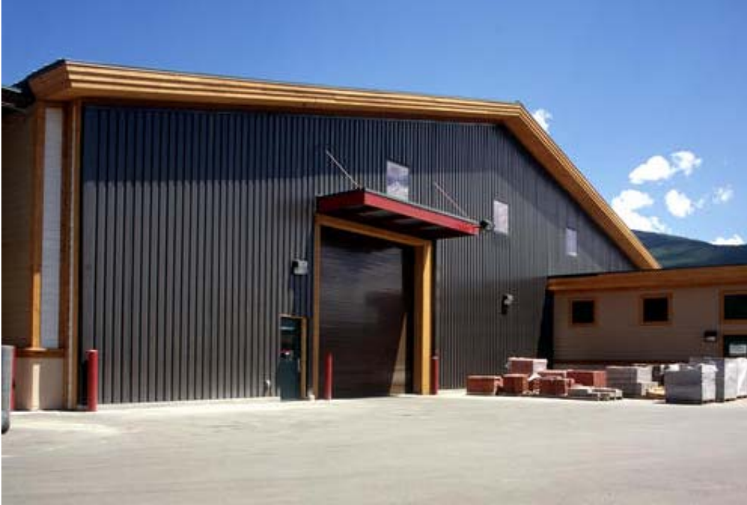
Figure 5-12 Transpired solar collector on the south wall of the warehouse
