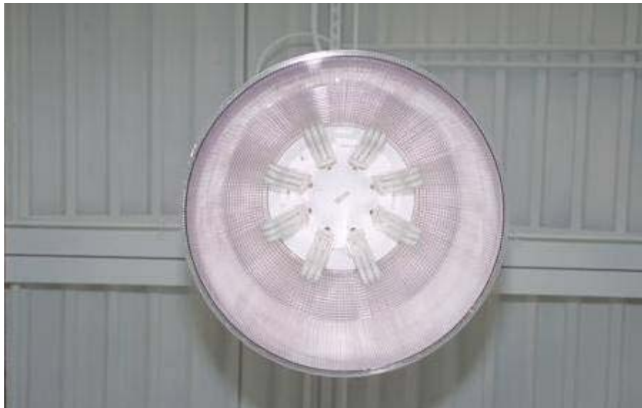
Figure 5-7 Pendant luminaire with eight 42-Watt CFL bulbs used in the retail and warehouse areas
