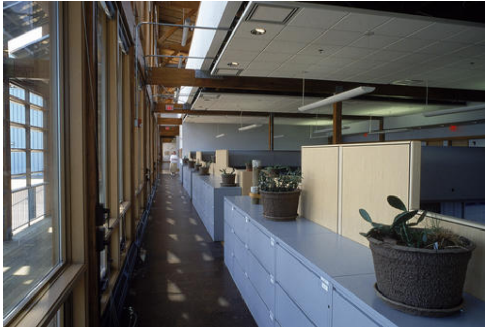
Figure 4-4 T-8 overhead lighting on the first floor (100% indirect)
