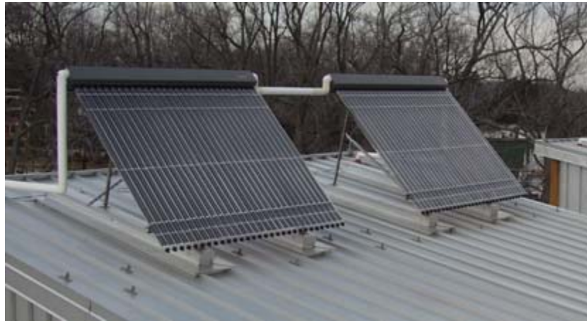
Figure 4-13 Evacuated-tube solar collector arrays
