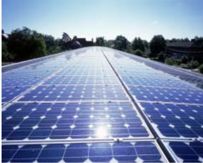
Figure 4-11 View of PV system from west end
