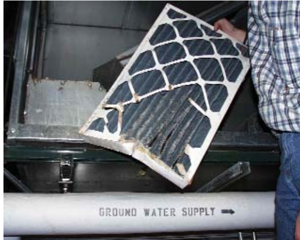
Figure 6-5 Damaged ERV filter
