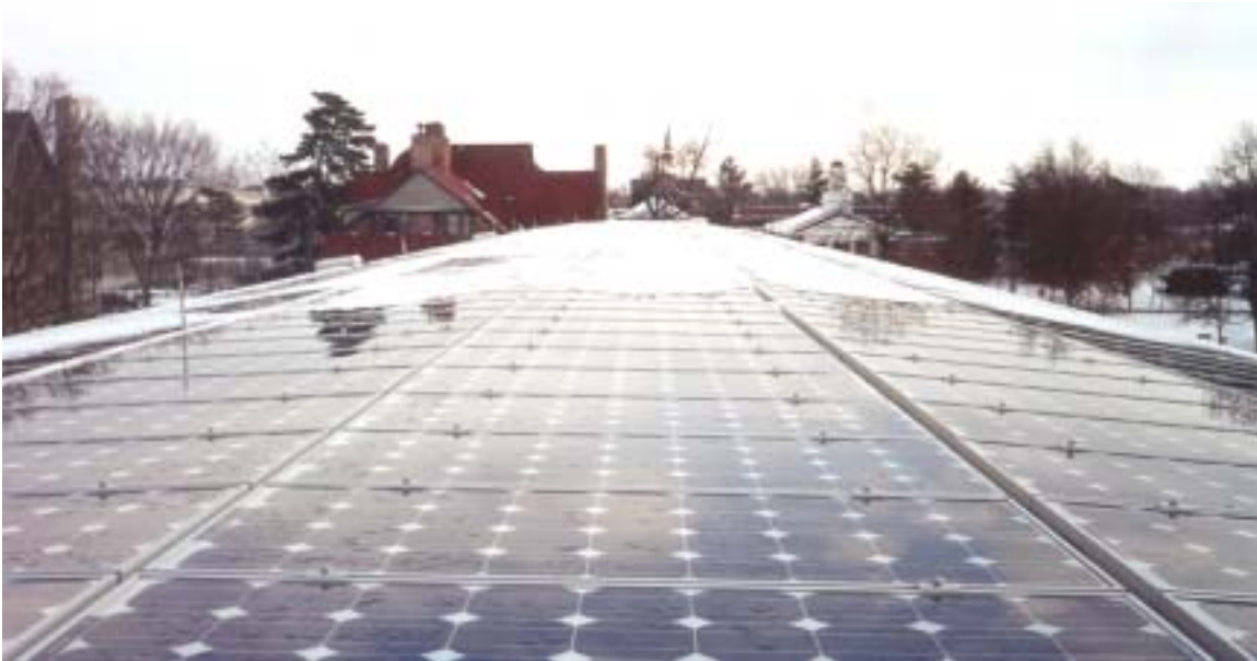
Figure 6-19 PV array partially covered with snow
