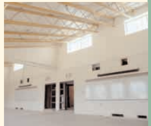
Clerestory windows allow light into a classroom (above). A curved sunshade wall shades the school's glass corridor along the front of the school (left).
