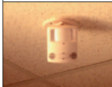
Daylight sensors combined with occupancy sensors are used as an energy-saving measure to turn the lights off if the natural light level is sufficient or if the space is unoccupied.
