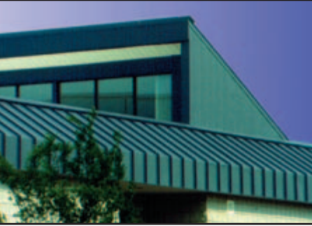
Using roof monitors to optimize solar access can significantly lower costs by reducing lighting and cooling needs.
