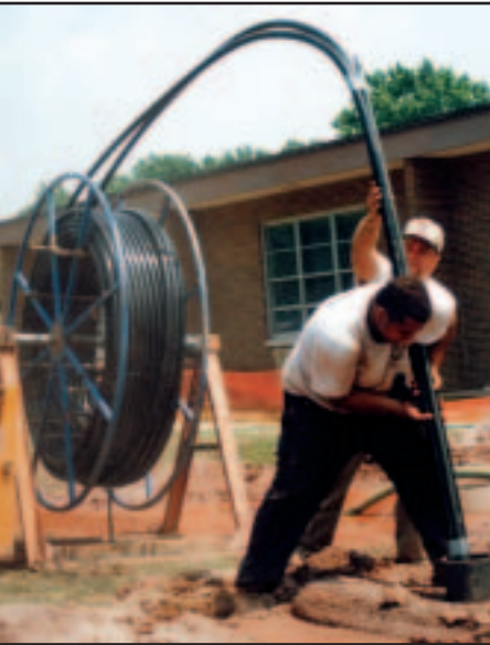
Photo: Advanced Energy
