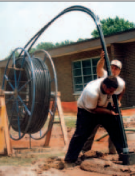
Photo: Advanced Energy
