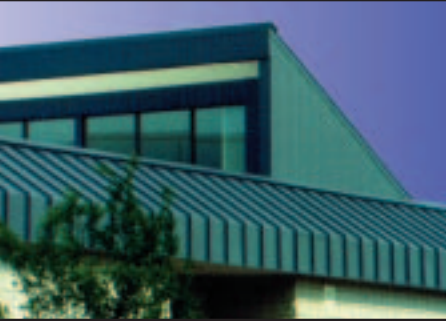
Clear double glazing has to be used to optimize solar access. Overhangs block excessive radiation in the warmer months.
