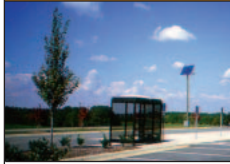
These stand-alone photovoltaic systems power parking lights.
