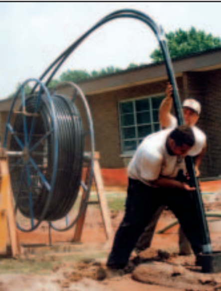
Photo: Advanced Energy
