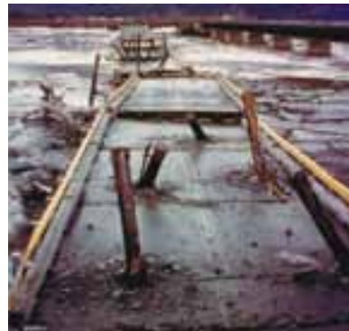
Remains of highway bridge, Portage. Wooden pilings pierce deck they used to support. Aerial view, p. 14.
