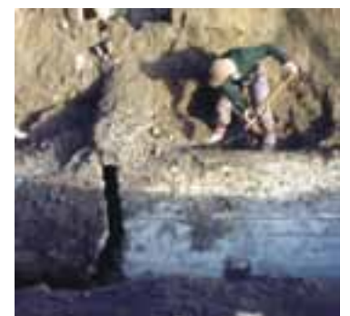
Broken sewer main, Puerto Montt.
