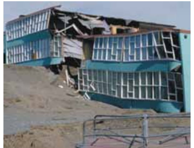
School torn by landslide, Anchorage.
