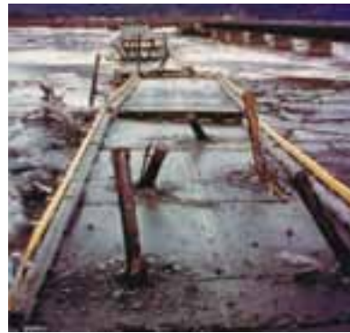
Remains of highway bridge, Portage. Wooden pilings pierce deck they used to support. Aerial view, p. 14.
