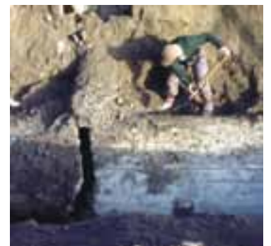
Broken sewer main, Puerto Montt.
