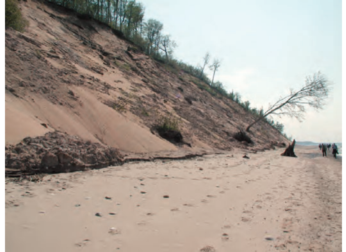
Figure 37. Failing bluff on the south shore of Lake Superior in Michigan, showing shallow slide of tree-and-root mat down sand slope that is at the angle of repose.
