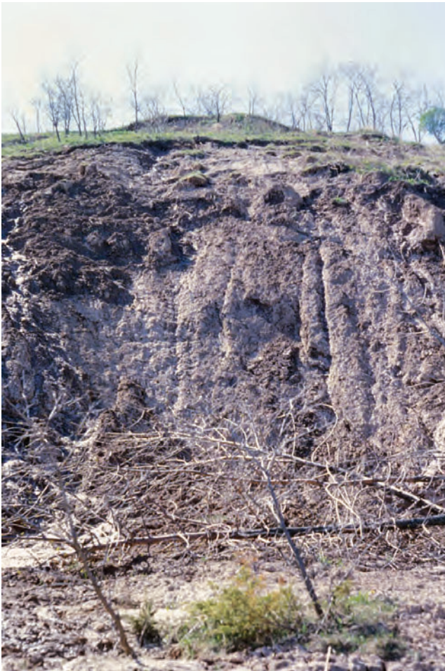
Figure 22. Western Lake Michigan bluff face in mid summer shows the effects of sheetwash and the development of gullies. These shallow gullies form every year on clayey till where solifluction and shallow slides occur in winter. From Sterrett (1980).
