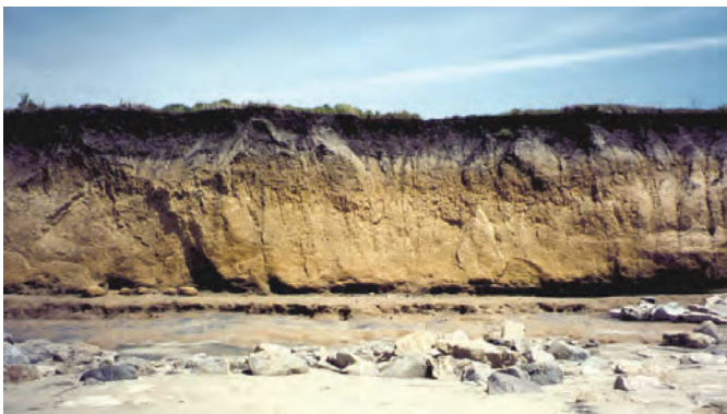
Figure 27. Ground-water discharge at the base of a coastal cliff in northern San Mateo County, California, that is underlain by impermeable rock has eroded a low notch, which undercuts and potentially destabilizes the cliff. Cliff is about 3 m high.
