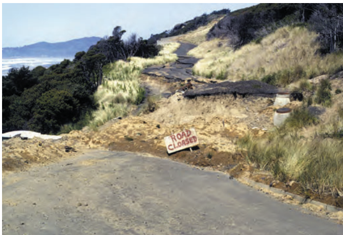
Figure 20. The disruption of streets and sewers in the Stratford Estates development north of Yaquina Head (fig. 5), resulting from a slowly moving landslide. (From Komar, 1997.)
