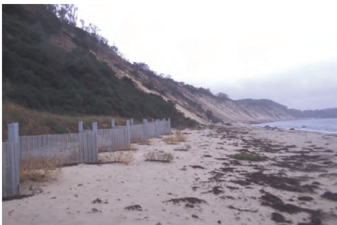
Figure 21. Bluff of outwash sand and gravel at the White Cliffs area of Plymouth, Mass., have historically eroded at rates between 1m/yr and 2 m/yr (James O’Connell, Woods Hole Sea Grant, oral commun., 2002). The gabion wall was built prior to laws prohibiting such structures to slow shoreline retreat.
