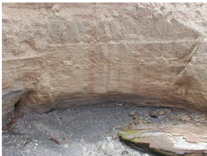
Figure 15. Wave-cut notch, approximately 3 m high, at the base of a sea cliff eroded into interbedded sandstone and shale at Cabrillo National Monument, San Diego County, California. The erosion is enhanced by the abrasive effect of the coarse beach sediment that is entrained within the waves. Notice the sea cave at the left side, where a steep fault cuts the strata.
