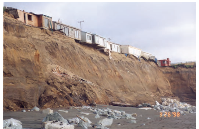
Figure 2. Rapid retreat of this sea cliff in Pacifica, California, caused damage to these houses, which later were declared unsafe and demolished. Compare with the cover photo of the same area, taken about 2-1/2 months previously, before the arrival of the 1997-98 El Niño storms.
