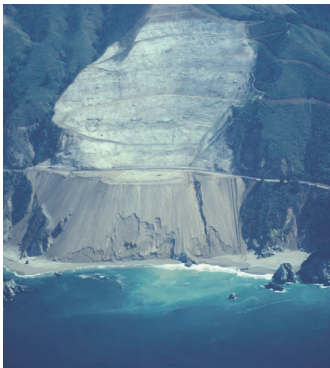
Figure 33. Reconstruction of California State Highway 1 along the Big Sur coast after a major coastal landslide in 1983. Total cost: $7,500,000.
