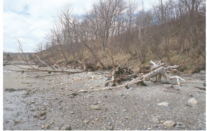
Figure 22. Erosion of glacial-marine mud bluffs in Rockland, Maine, proceeds relentlessly between large landslide events.
