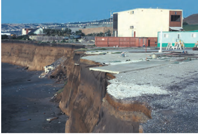
Figure 16. Erodible bluffs consisting of unconsolidated marine terrace deposits and soil in Pacifica; the site of previous mobile home pads that had to be abandoned because of sea-cliff retreat during the 1983 El Niño.
