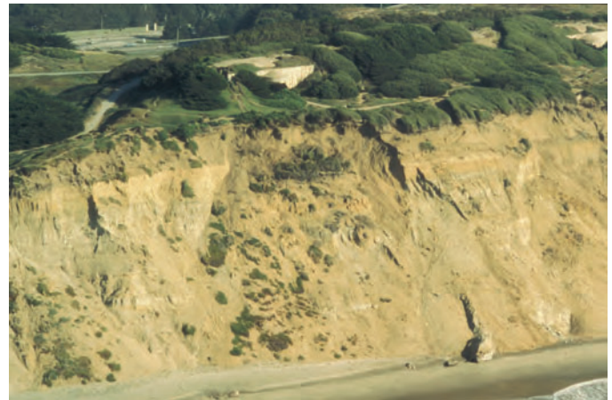
Figure 40. A shallow cliff failure on the upper part of a steep sea cliff in the San Francisco area of California, caused by seismic shaking during the 1989 Loma Prieta earthquake.
