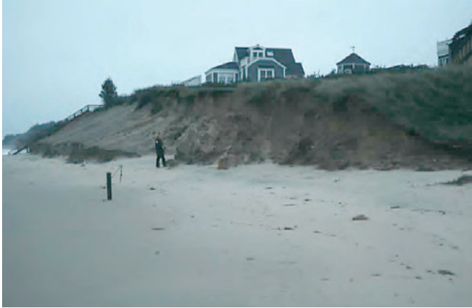
Figure 20. Bluff erosion on the south shore of Cape Cod, Mass. threatened condominiums during the “Halloween Storm” of 1991. The bluff retreated at least a meter at the beginning of the storm, and sand was dumped onto the beach to protect the buildings.
