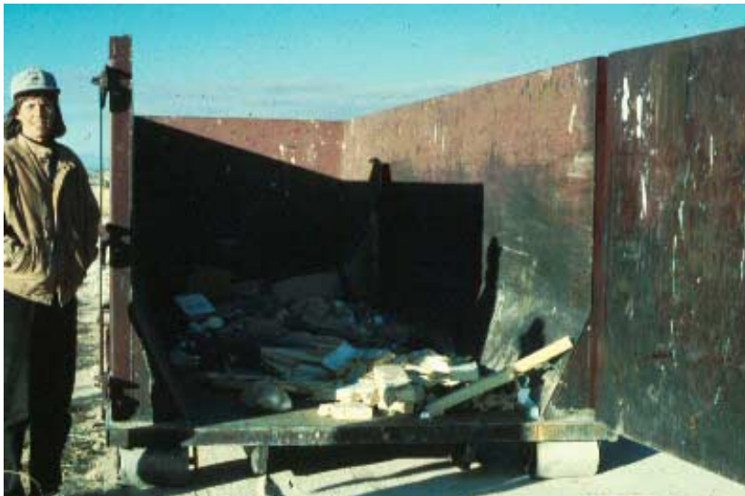
Figure 5. Dumpster with all construction waste including that from framing and drywall
