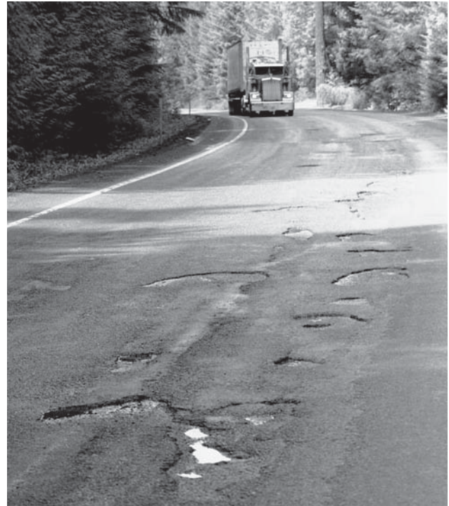
Oregon 58, a major freight route, east of Oakridge shows the signs of surface damage caused by harsh winter weather.
