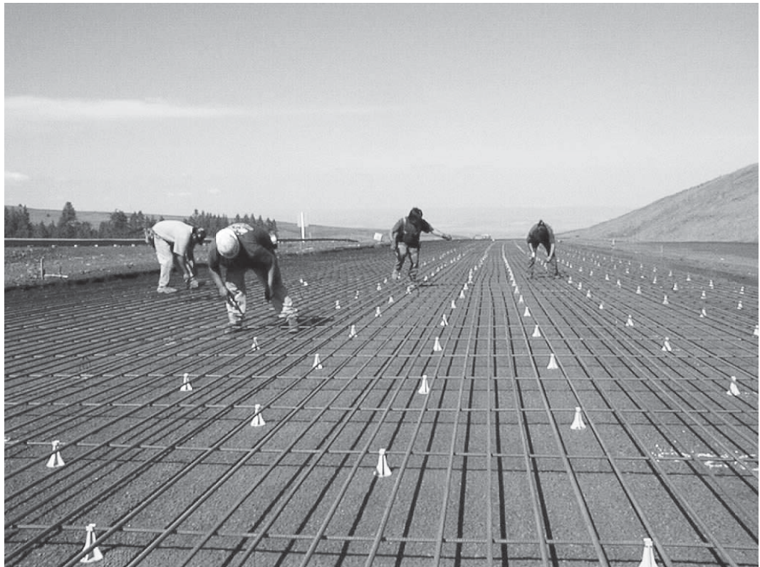
Crews are adding a lane to a segment of Interstate 84 on Emigrant Hill near Pendleton.
