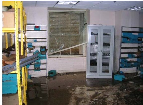
The floodwaters surrounding the IRS building broke through windows in several rooms in the basement of the IRS building. (Photo provided by the IRS)
